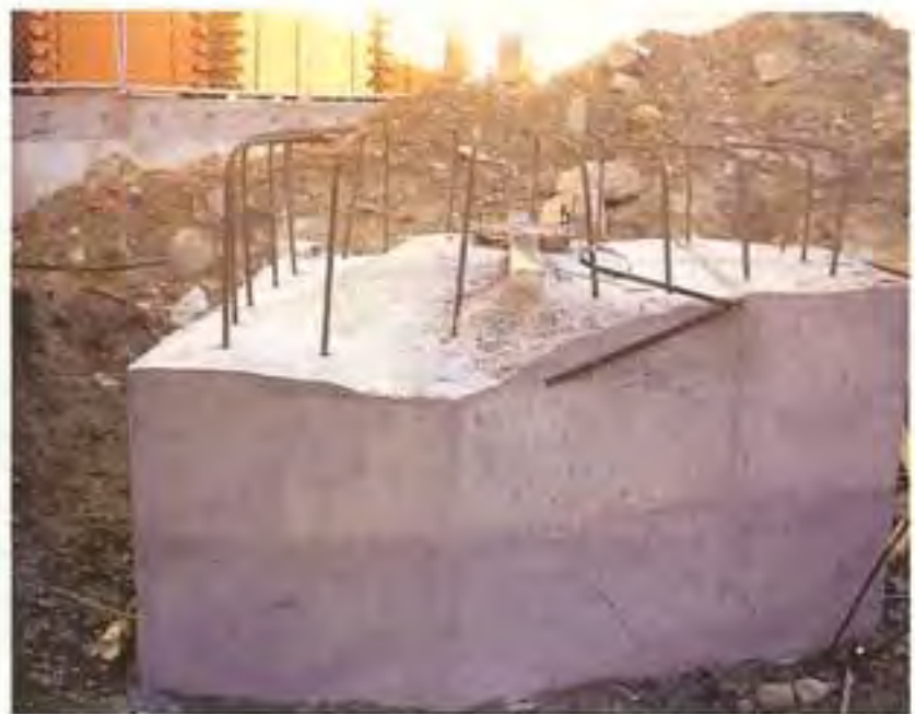
Without special inspections, construction errors that compromise structural integrity could easily be covered up, only to be revealed if and when a problem occurs. For example, the contractors ran out of concrete while casting this pile cap, but assured the inspectors that they would top it off with the next pour.
